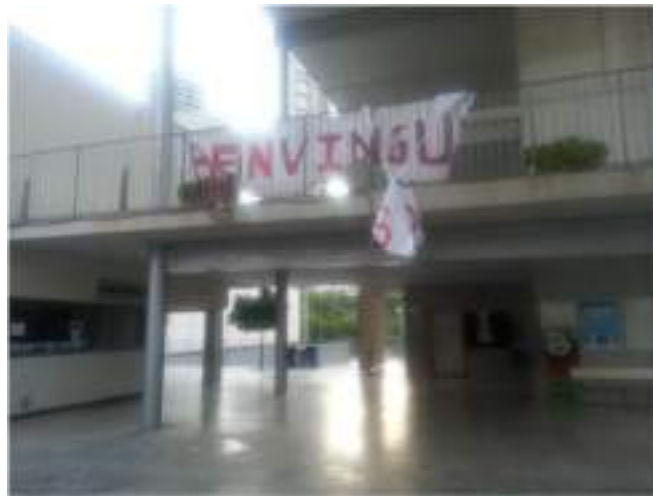
Figure 19. Entrance hall to an open-air design high school. Materials damaged by the wind.
